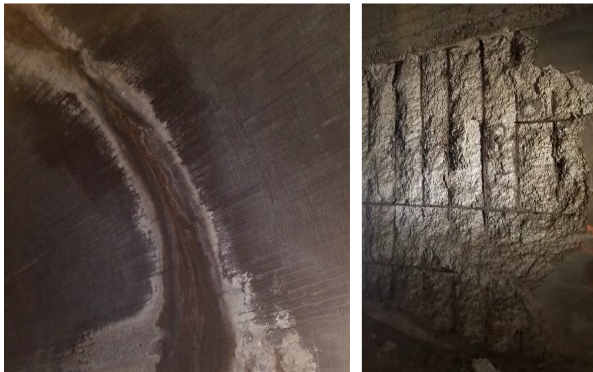
Figure 19: Severe deterioration and spalling of concrete
