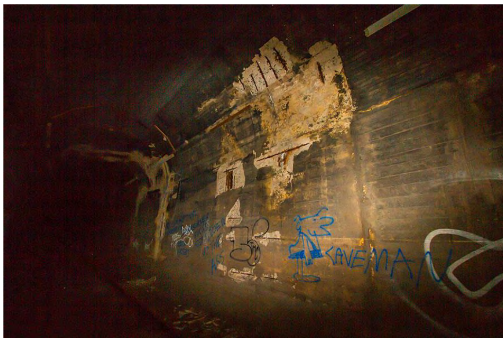
Figure 4: Scraped wall potentially due to accident of 1971
